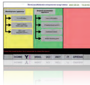
electrical components status
